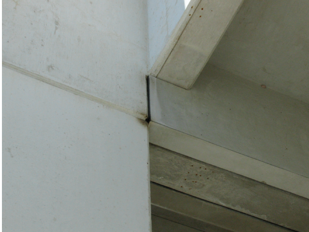
Figure 1: Notice the dark smudge at the bottom of the seam.
